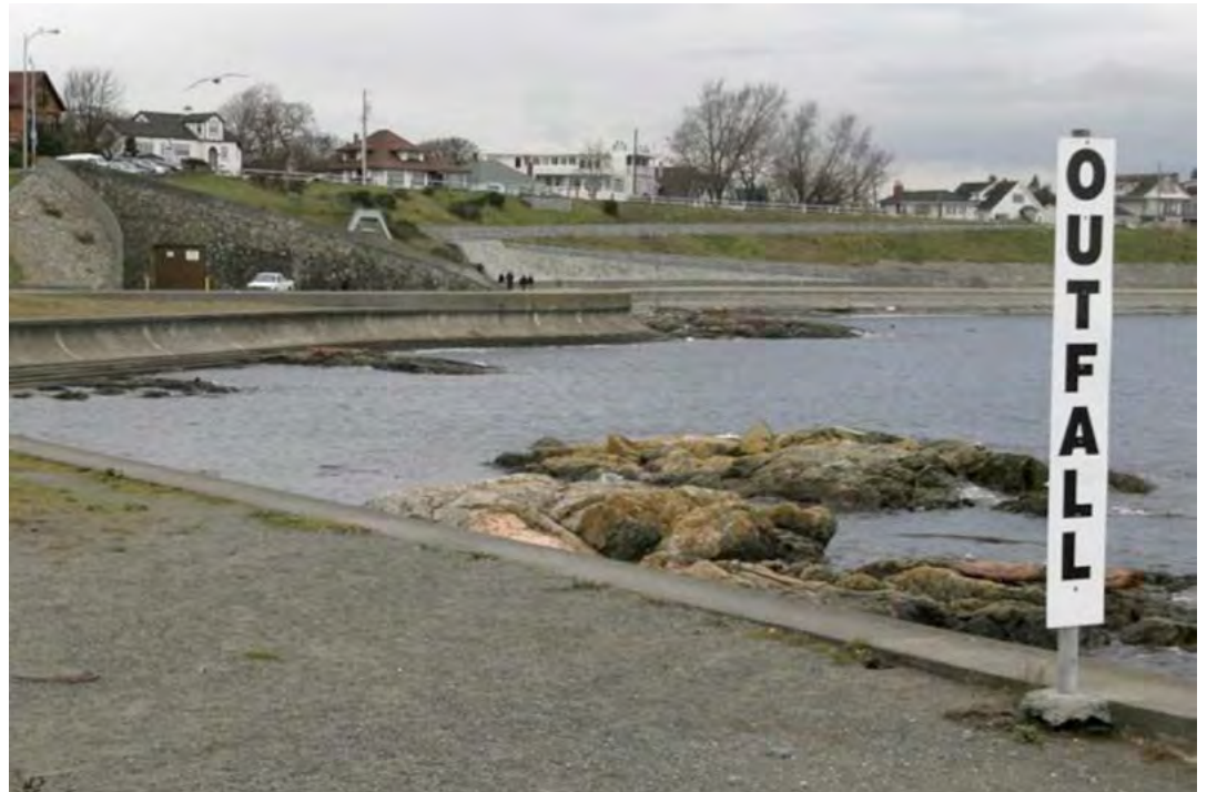
Sewage outfall at Clover Point, Victoria, BC
